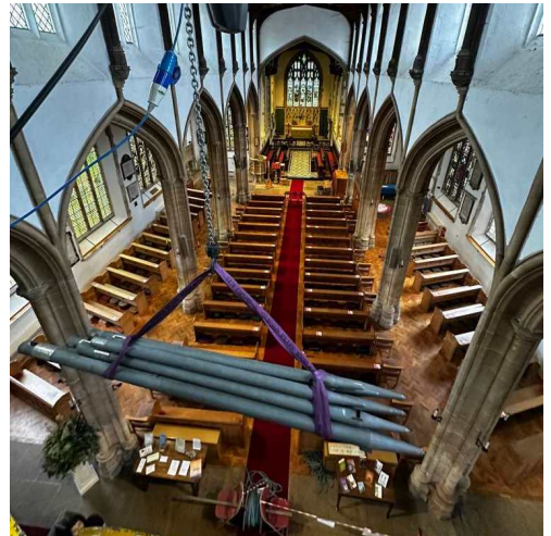
Looking down the Aisle from the platform with a load of pipes ready to be lowered to the floor.
