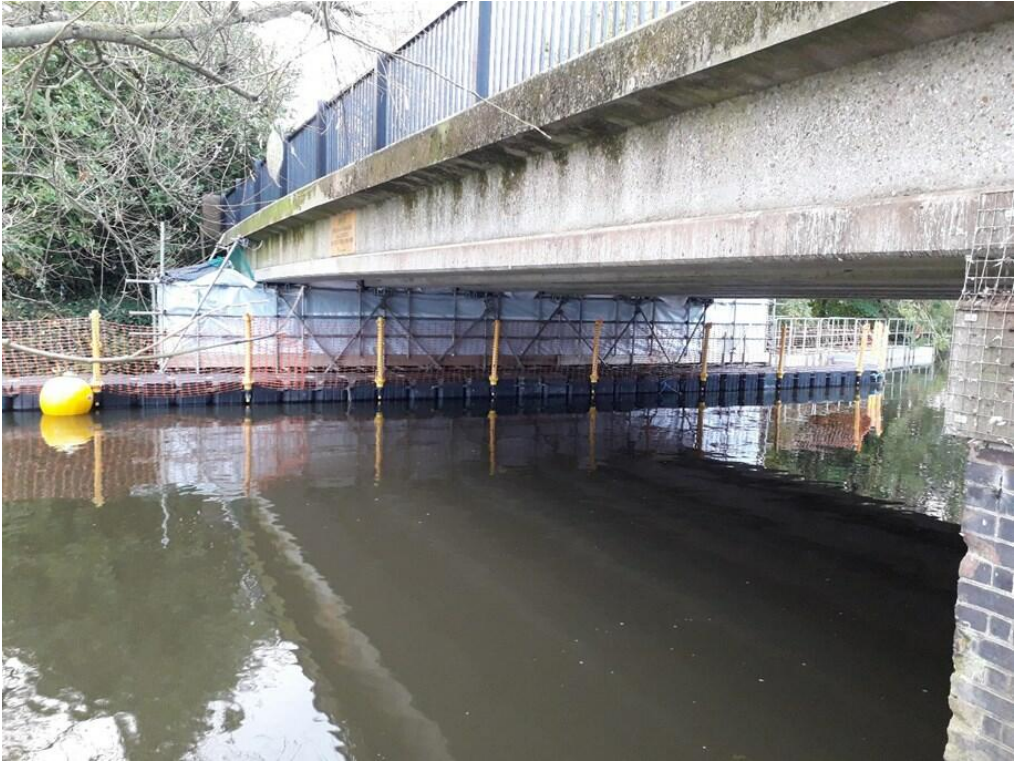
Temporary scaffolding installed adjacent to South abutment to provide access to bearings.
