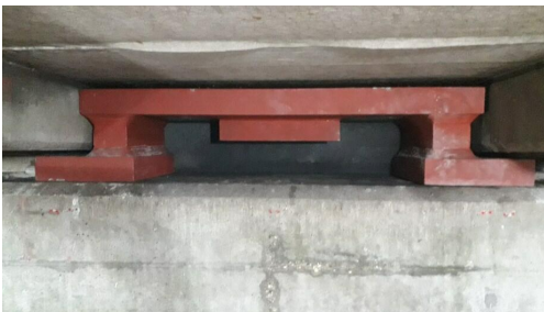
Corroded existing bearing supporting bridge beam and cracked concrete abutment.
